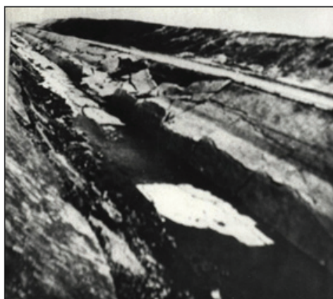
Figure 1. Example of disorders in the construction of the “Samour –Apcheron” concrete channel.
