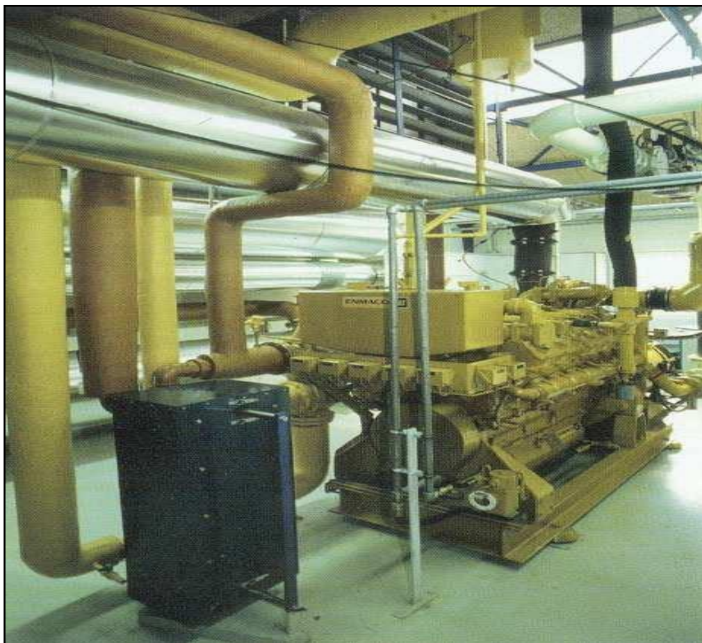
Figure 4.36: turbine à gaz. [49]
