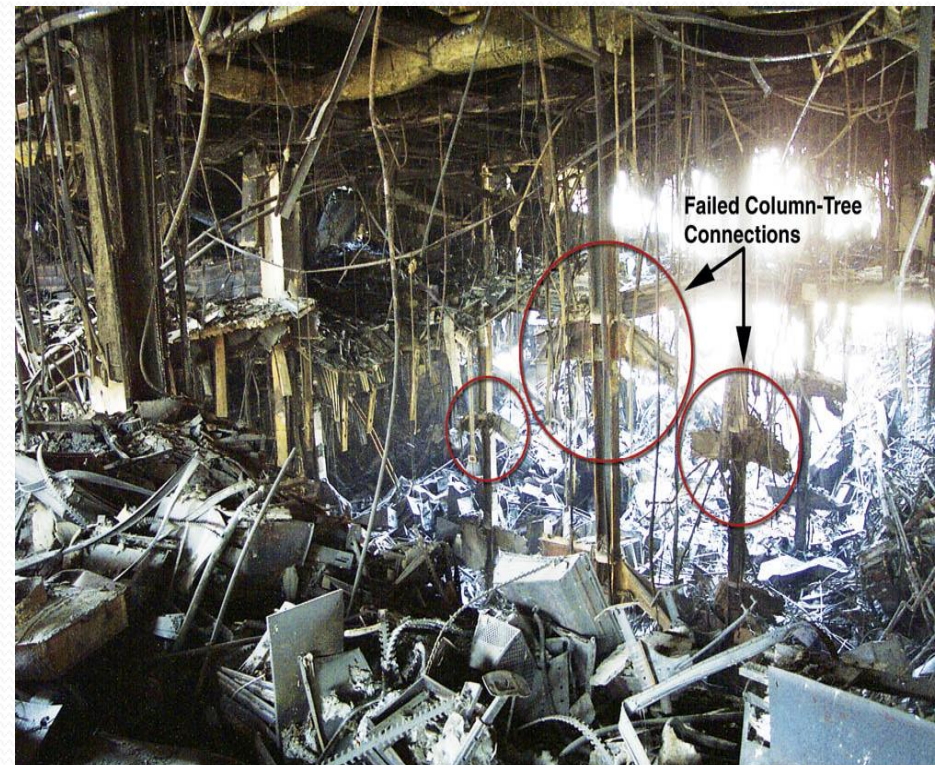
Partial Connection and Floor Failures in WTC 5
